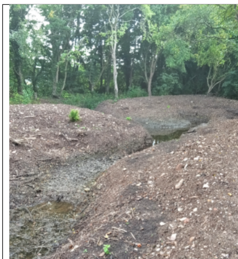
Figure 14: A newly constructed storage pond at Padgets Lane, Redditch. To add ecological value it was designed to permanently hold water at low levels. (Annex A, Table A1, item C7 refers.)
